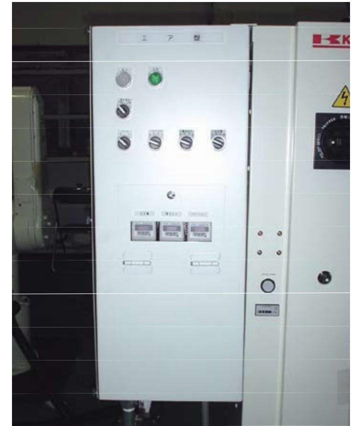
Painting unit control panel
